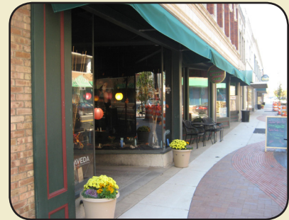
The sidewalk is taking shape along Michigan Avenue. The bricks are intended to mimic the movement of the river, as selected by Battle Creek citizens during the public input process.
